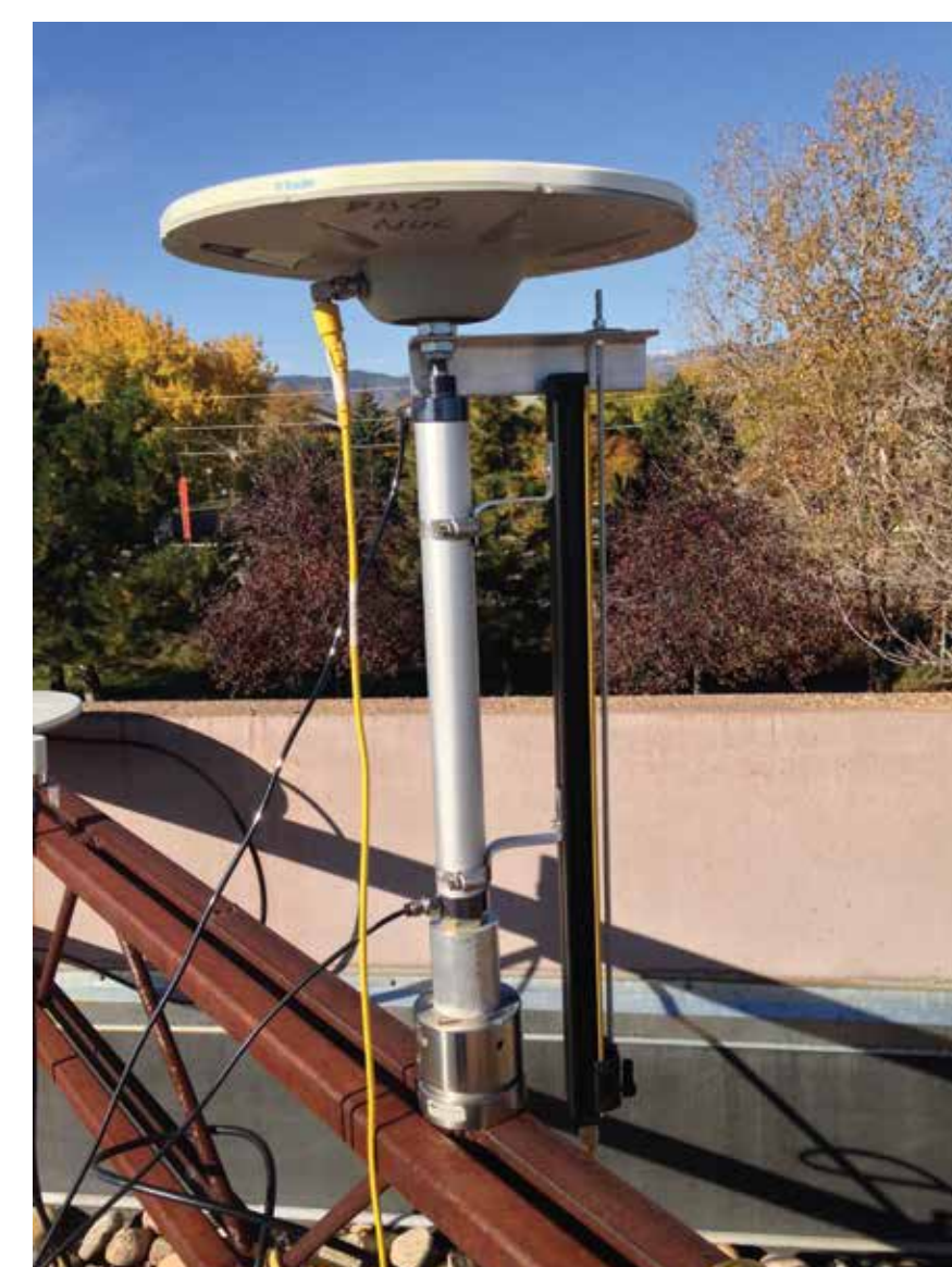
A close up of the pneumatic cylinder, linear position sensor and Trimble Zephyr antenna.
